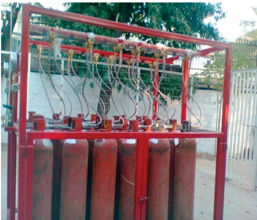
Figure 7.21 Cylinder bank/cascade installed at the hydrogen fueling station.
